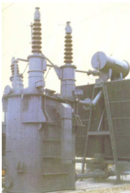
Rys. 6.3.6. Transformator 15 MVA, 132/25 kV
